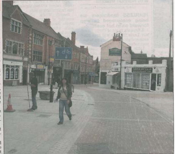
NEARLY DONE - work to finish off Kettering's Market Place nears completion ET picture by Alison Bagley 05-10-11-AB-5-23
